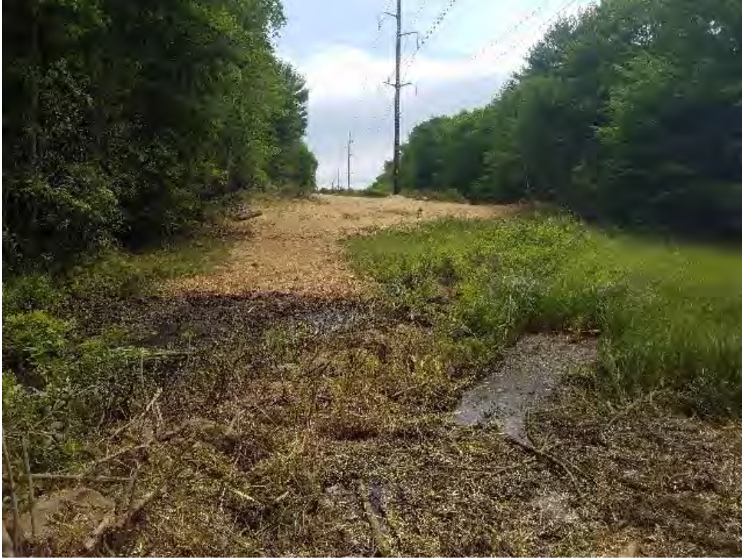
Fig 19: Timber mat bridge removed at stonewall WP-28 and through wetland DW25. Viewing east. (06-03-20).
