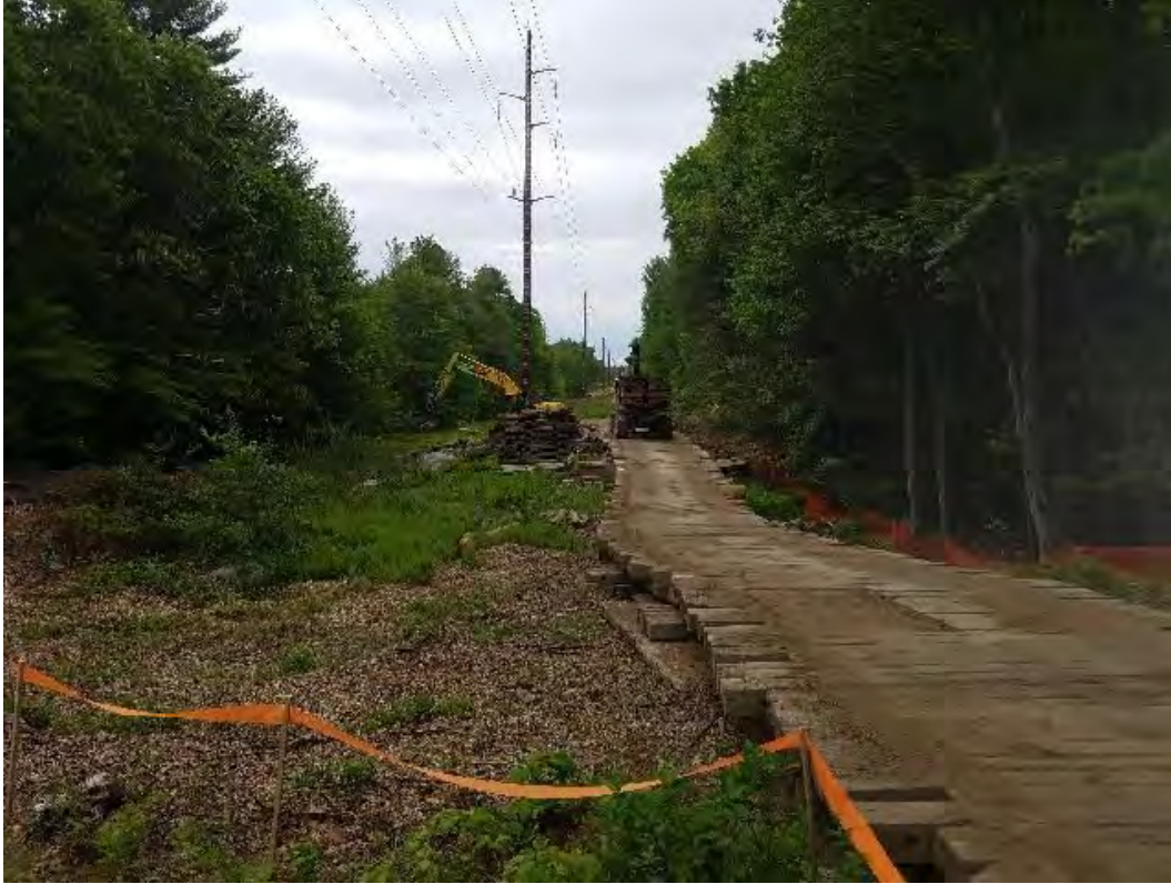
Fig 15: Removing timber mat access road and work pad at Str. 89. Viewing southeast. (06-03-20).
