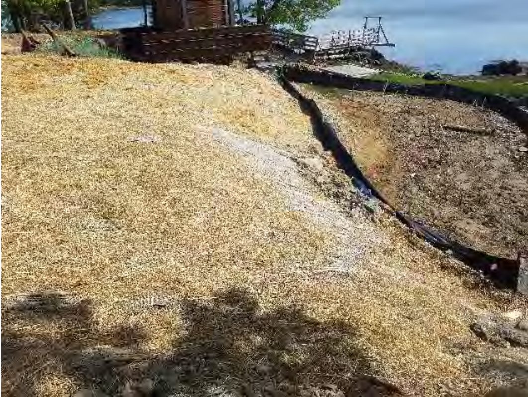
Fig 3: Toe of slope BMPs and salt marsh restoration at Getchell property/west side of the Bay. Viewing north. (05-28-20).
