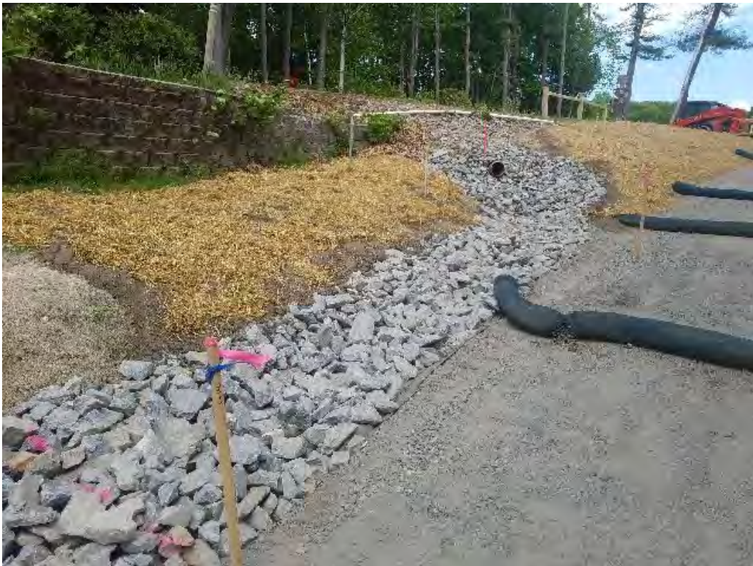
Fig 10: Rip rap swale installed along the slope at Gundalow landing/east side of the Bay. Viewing east. (05-29-20).
