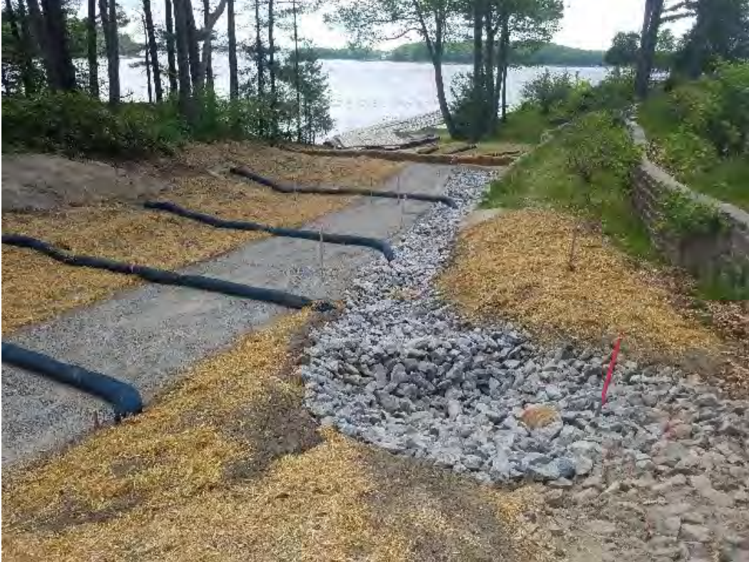
Fig 9: Rip rap swale installed along the slope at Gundalow landing/east side of the Bay. Viewing southwest. (05-29-20).
